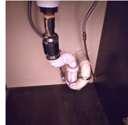
Active leak below a bathroom vanity
