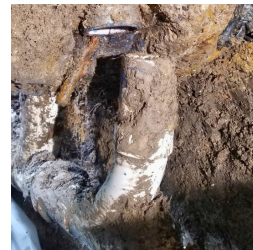
Broken sewer piping exposed below a slab
